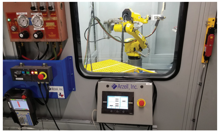
Electrical control valve system
